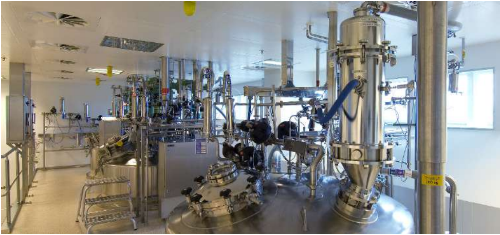
Fig. 14a. Production of solutions and temporary storage
