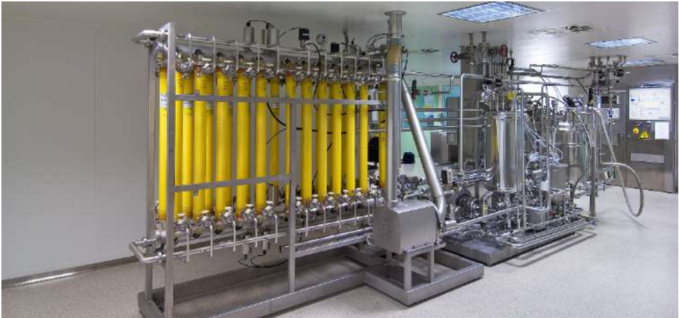
Fig. 14b. Ultrafiltration facility
